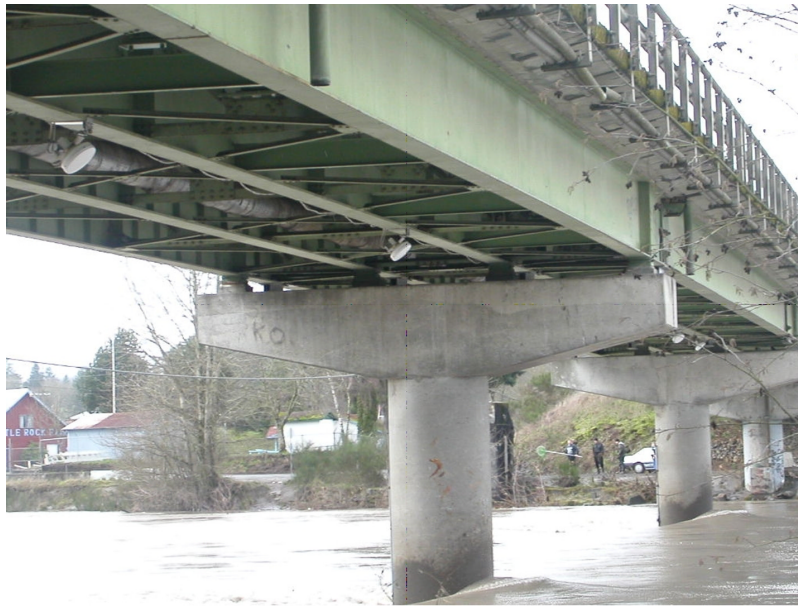
Figure 7. View under Cowlitz River bridge with four of eight RiverScat antennas visible and pointing upstream.
