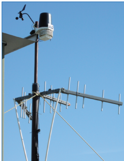
(Left) The RiverSonde antenna mast. Three 0.5-meter Yagi antennas are arranged symmetrically in a tight sector. A weather station atop the antenna mast provides wind and meteorological data.
