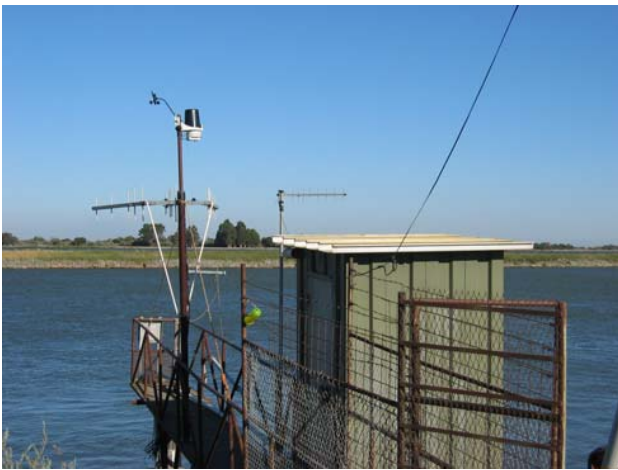
Fig. 8. RiverSonde installation at Threemile Slough. The RiverSonde antenna is mounted on the left side of the walkway and is over the water about 4 m from the bank. The weather station sensors are above the antenna. The smaller antenna is for USGS data telemetry. The USGS and RiverSonde equipment are inside the shelter.
