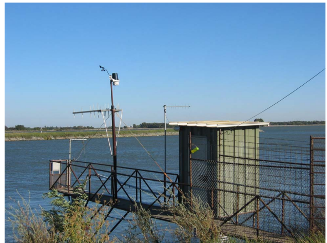
Fig. 1. RiverSonde installation at Threemile Slough. The RiverSonde antenna is mounted on the left side of the walkway and is over the water about 4 m from the bank. The weather station sensors are above the antenna. The smaller antenna is for USGS data telemetry. The USGS and RiverSonde equipment are inside the shelter.
